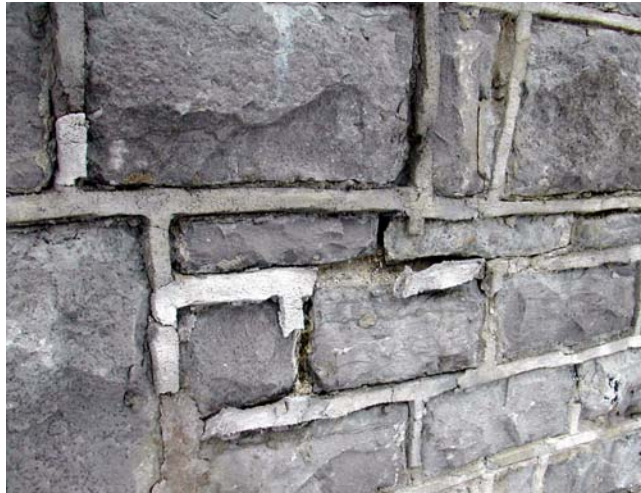
Figure 1 Frost damage in a wall with a dense repointing mortar
